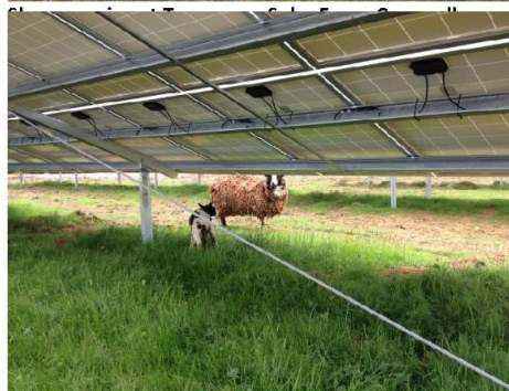
Lamb underneath array at Newlands Solar Farm, Devon
