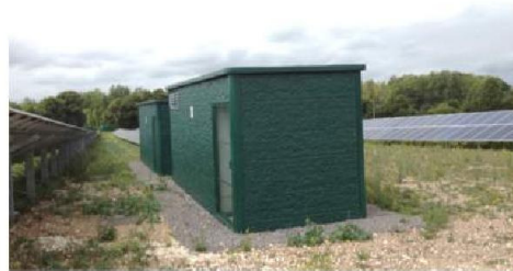
Inverter Building, Hatchlands Solar Farm, Devon
