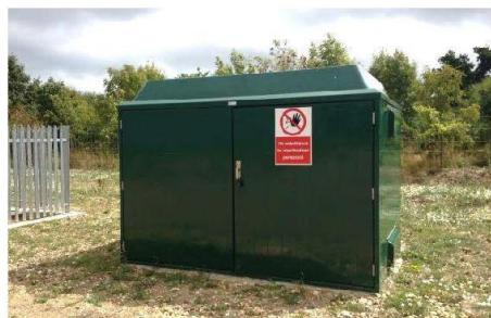
Customer Substation, Tavells Farm, Hampshire
