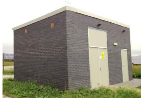
DNO Substation, Little Trevease Cornwall
