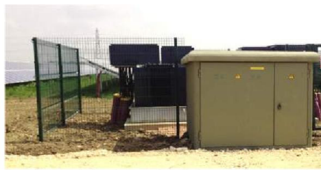
Transformer in background, switchgear in foreground.
